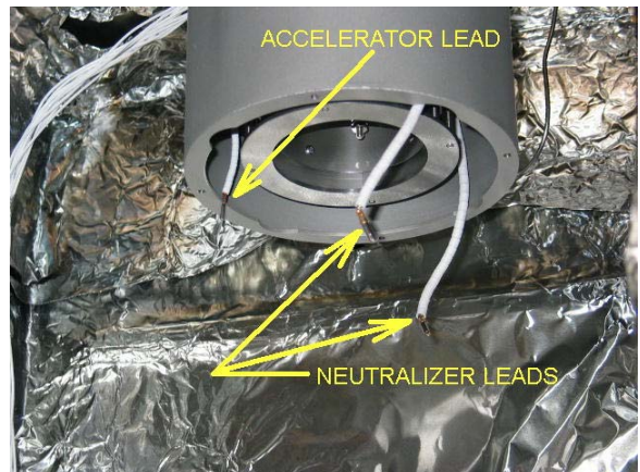
Picture 4.25. Electrical leads.
